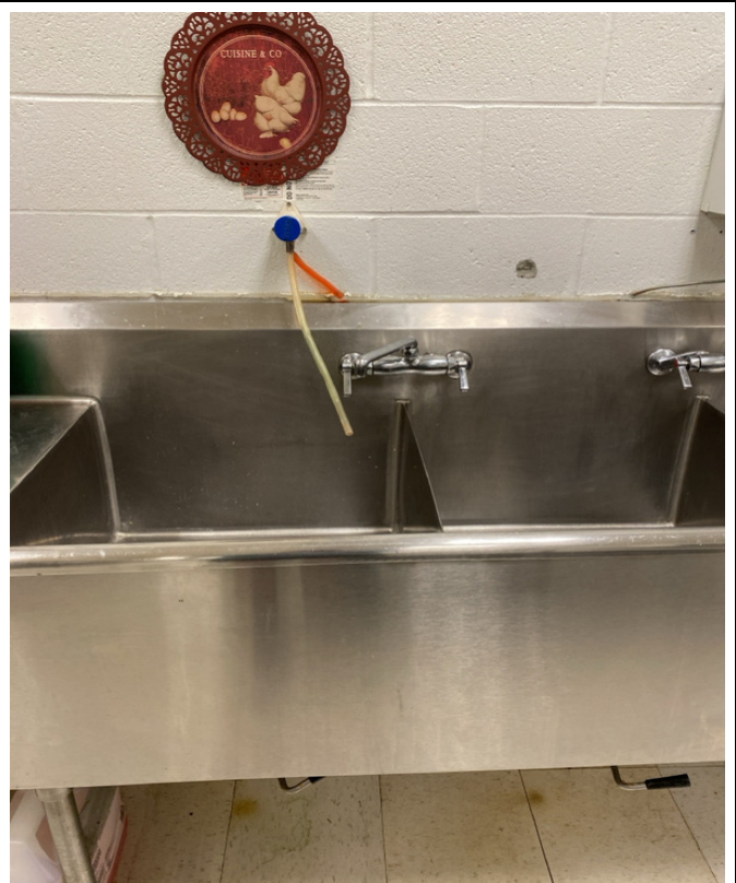
2/6/2024 - 327-8 - Elementary School - Kitchen - Three Bay Sink - Left
