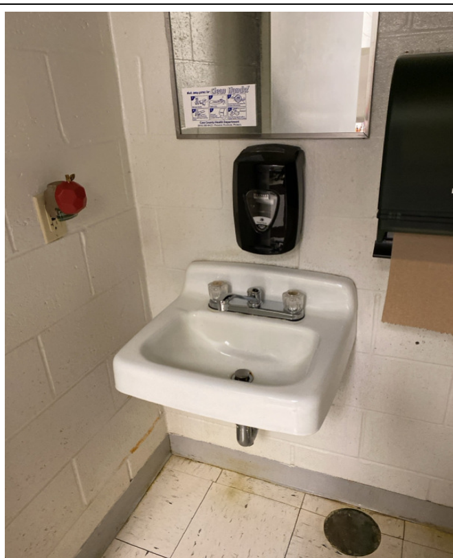
2/6/2024 - 327-10 - Elementary School - Kitchen - Restroom Sink
