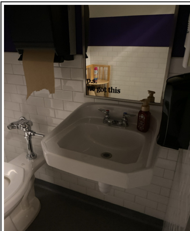
2/6/2024 - 327-25 - Elementary School - Room 38 - Left Restroom
