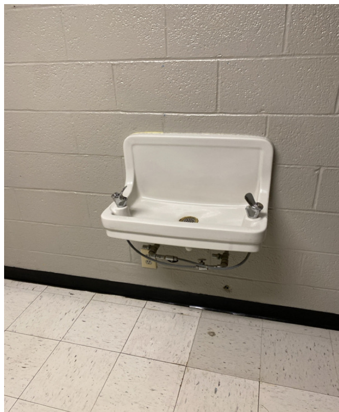
2/6/2024 - 327-19 - Elementary School - Hallway Outside Library - Out of Order
