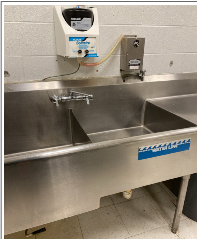
2/6/2024 - 327-9 - Elementary School - Kitchen - Three Bay Sink - Right
